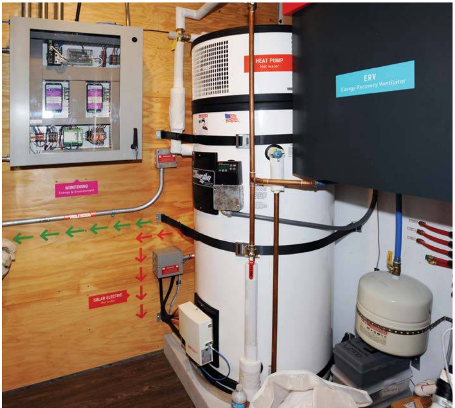
If you're in a climate where temperatures are 40°–90°F all year, consider a heat pump water heater to cut water heating costs by 50%.
